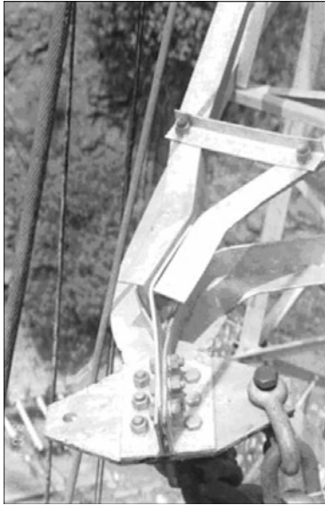
TEST – Failure of Cross Arm Tip
